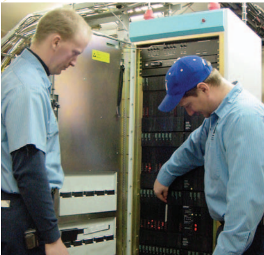
Adam Nelson and Joel Schmidt, two of Northwest's dedicated employees, inspect one of the digital switches.
